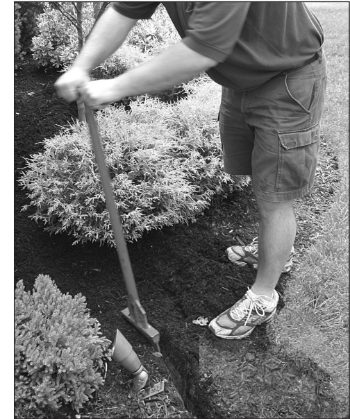
Pushing the tool back and forth widens the trench and creates a channel for the wire.
