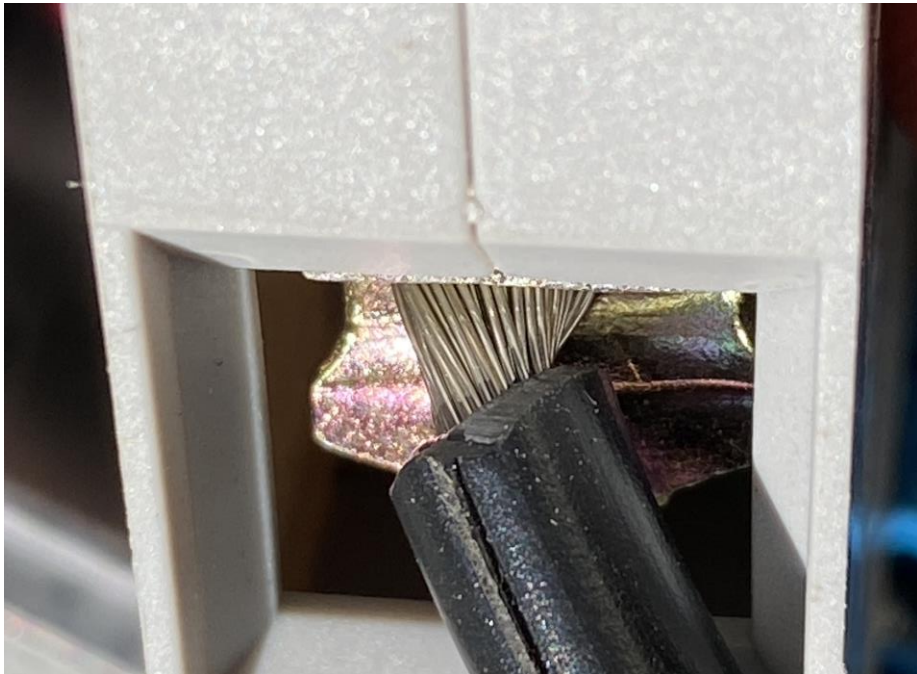
Example of a Solid Terminal Block Connection.
