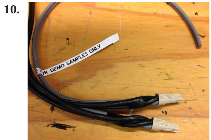
Wire Nut connections can never be used for outdoor splices. Use only for temporary electrical connections, such as product demonstrations.
